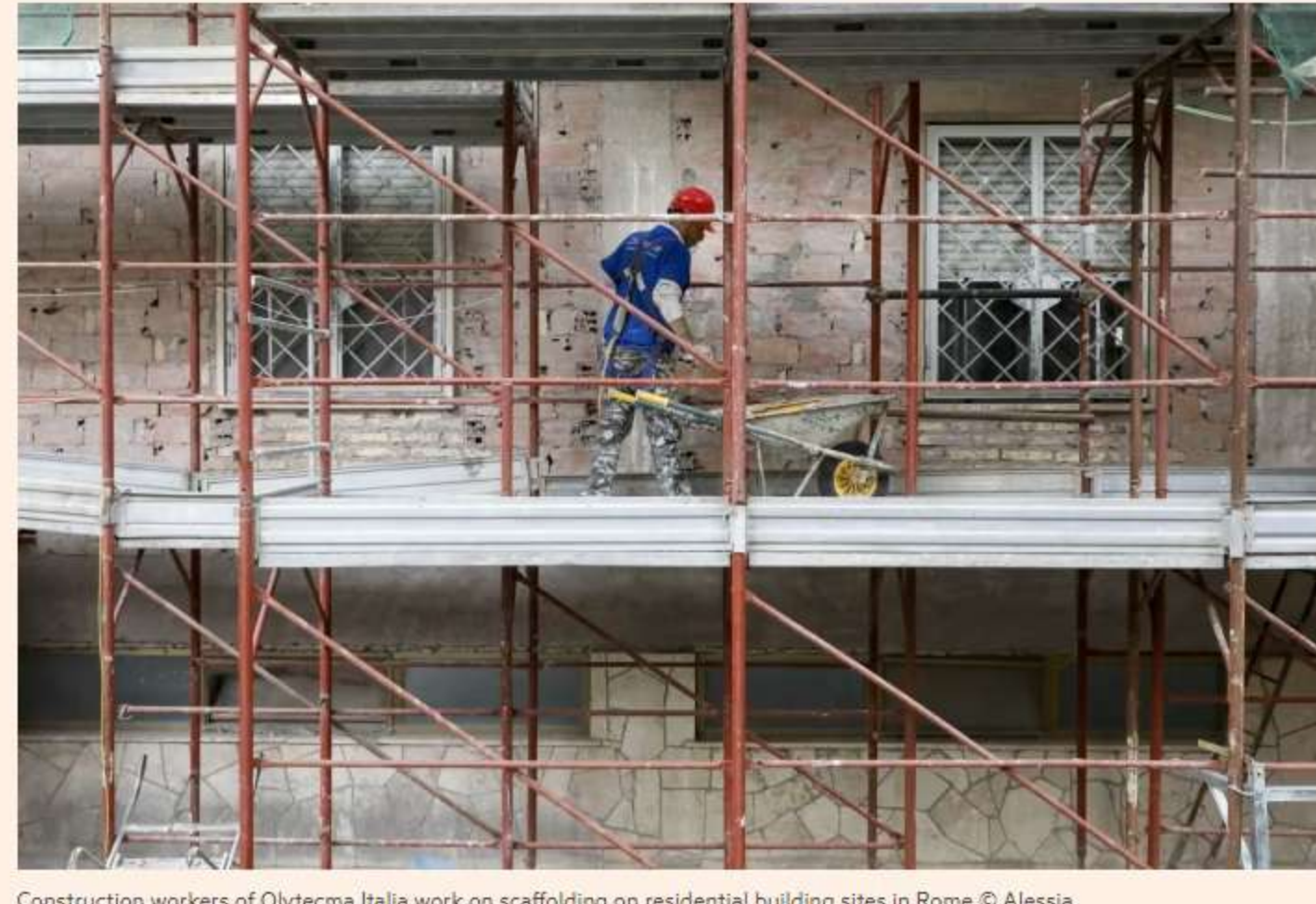
Construction workers of Glytecm Italia work on scaffolding on residential building sites in Rome © Alessia Pierdomenico/Bloomberg
